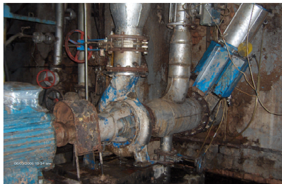
Fig. 1 – Liquor supply pump.
